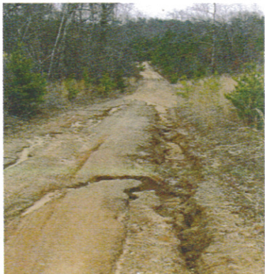
Abandoned Dirt Pits, Abandoned Surface Mines, and Access Roads that Need Stabilization
