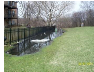
Drainage way is clogged by illegal dumping
