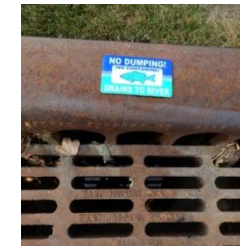
Storm Drain Medallion "No Dumping – Drains to River"
