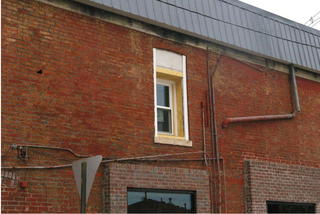
Figure 52. The historic window was removed and a smaller vinyl window installed in the window opening above. The window was inset from the main body of the building as well. This treatment is not permitted. See Guideline 5.5.1, 5.3.2, and 5.3.7.
