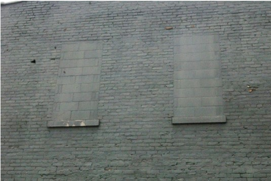
Figure 53. The historic window openings were blocked-in with concrete block on this building. This treatment is not permitted. See Guidelines 5.5.2 and 5.5.3.
