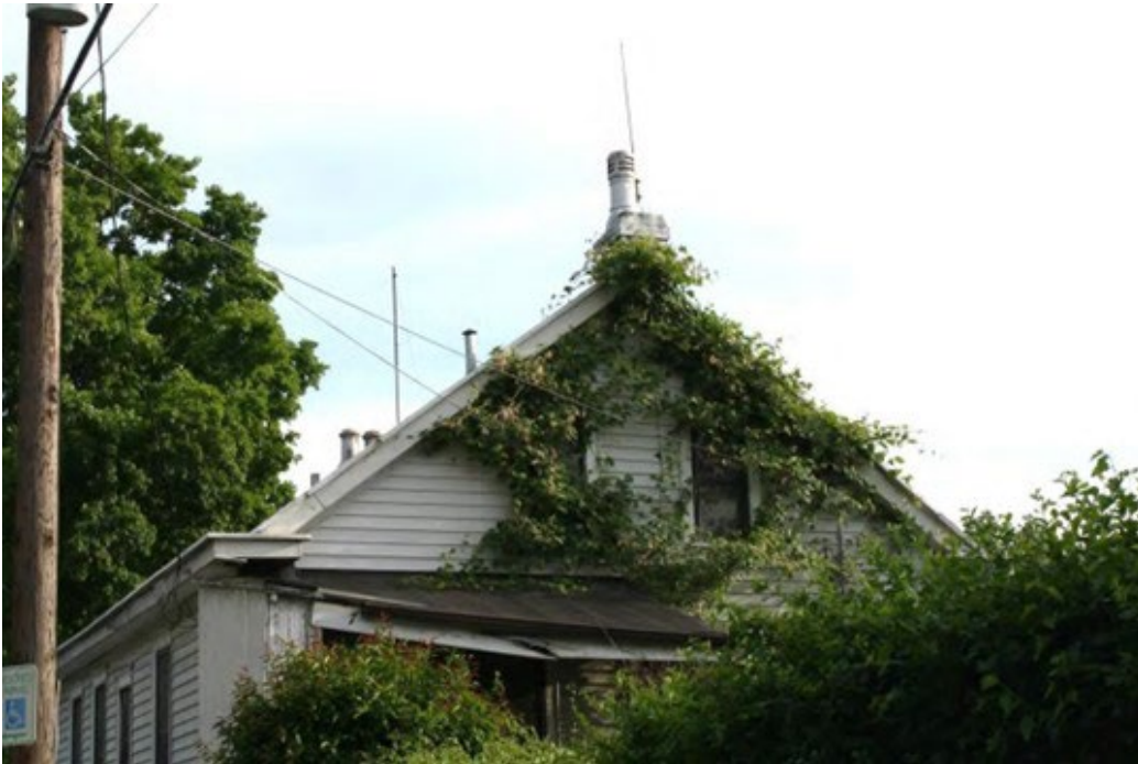
Figure 7. Ivy and other climbing plantings can be very destructive to historic buildings. See Guideline 1.2.5.
