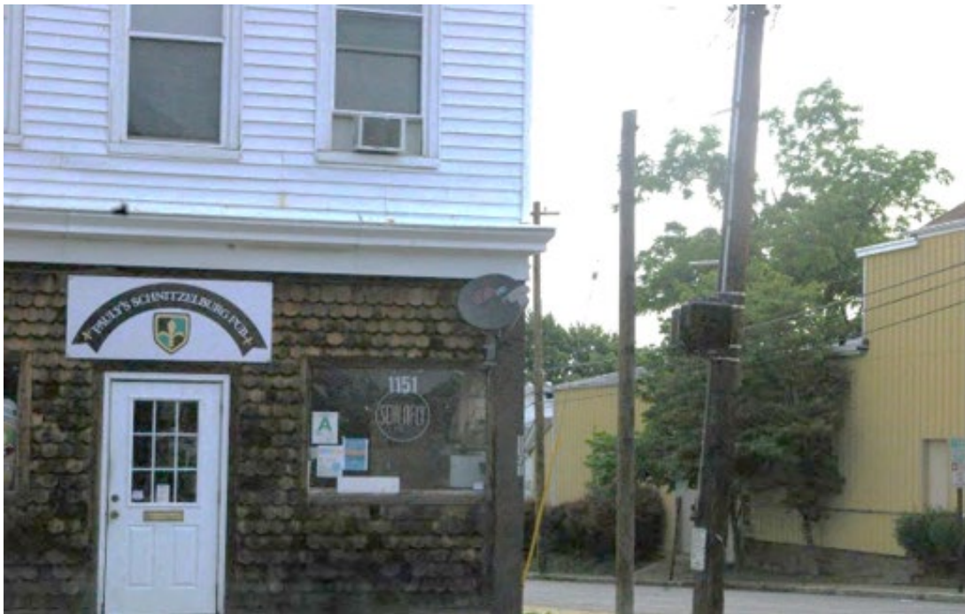
Figure 81. The window air conditioning unit on this building is placed on a street-visible façade. This treatment is not permitted under Guideline 9.2.1. In addition, a satellite dish is also appended to the building's primary façade, violating Guideline 9.4.1.
