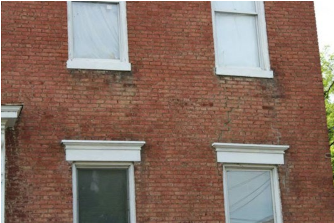
Figure 29. This street-visible brick patch was cleaned inappropriately, and the color wash removed. See Guideline 3.2.1.
