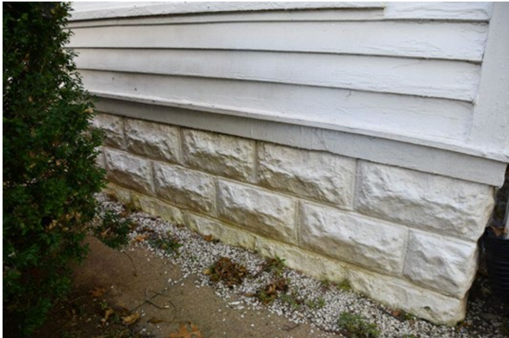
Figure 19. Molded concrete block foundation walls were occasionally used on early 20th century houses in the district. See Guideline 2.1.
