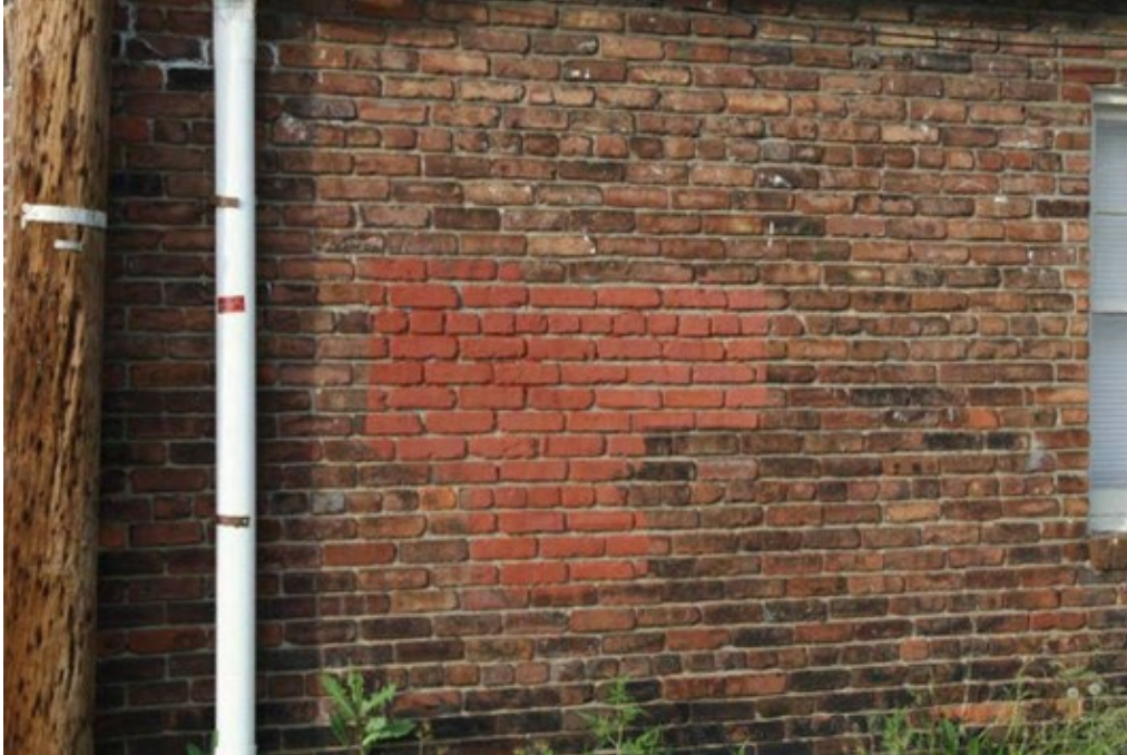
Figure 24. This brick wall needs repair and maintenance. Note the cracking along the wall and the missing mortar joints. See Guideline 3.1.2.
