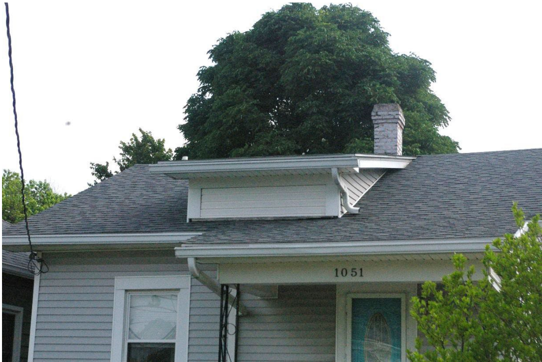
Figure 50. This dormer window was enclosed with vinyl siding. The original window likely remains intact. This treatment is not permitted under Guideline 5.5.2.
