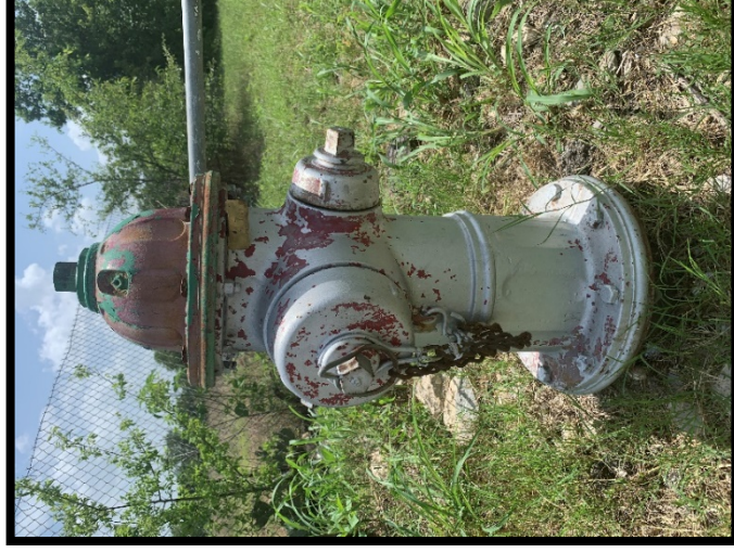
Fire Hydrants – Clear Vegetation and Repaint
