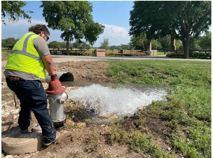
Public Works employee manually flushes fire hydrant which helps assure water quality. Hydrants are flushed monthly throughout the city.
