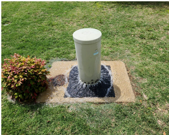
Automatic flush assemblies are used throughout the city to assure water delivered to customers is the highest quality. The flush assemblies are programmed to operate at various times of the day and night.
