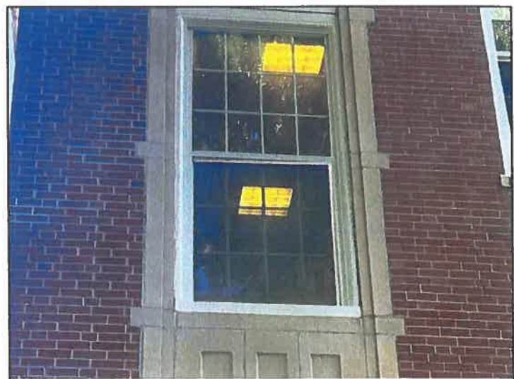
Photograph 2 – Window Concrete Deterioration
