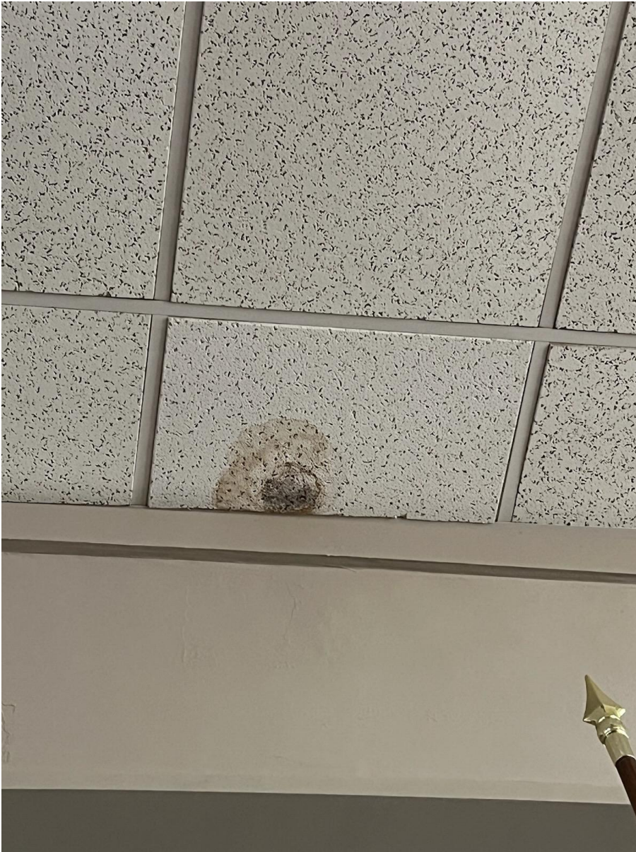
3 rd Floor Auditorium, active leak this one is now turning black.
