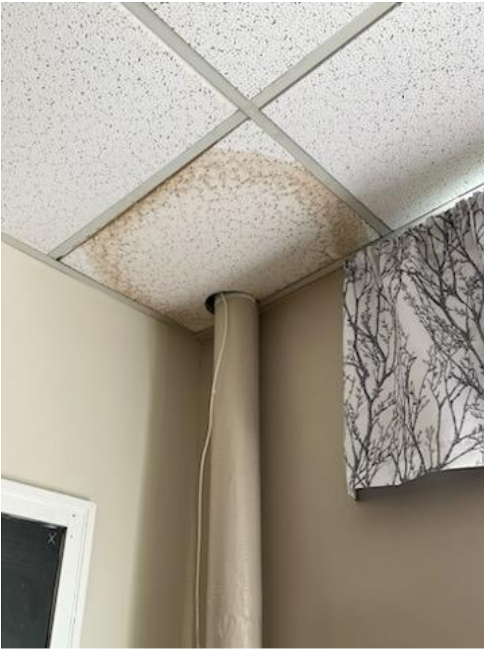
Code Enforcement Office has an active leak.
