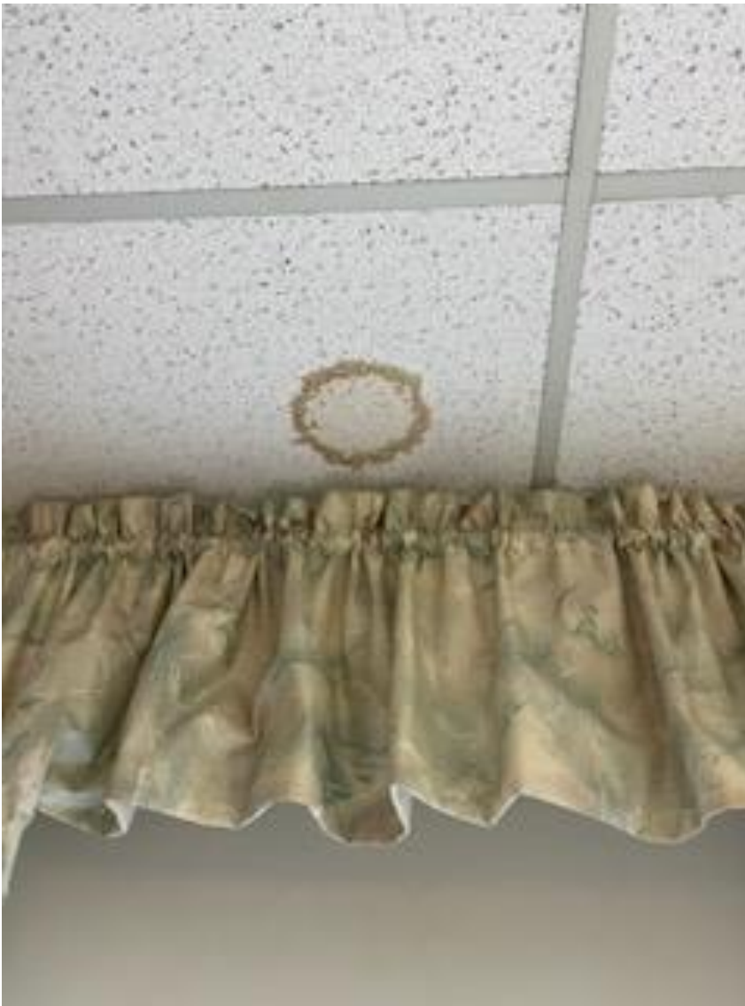
Clerk's Office, has an active leak.
