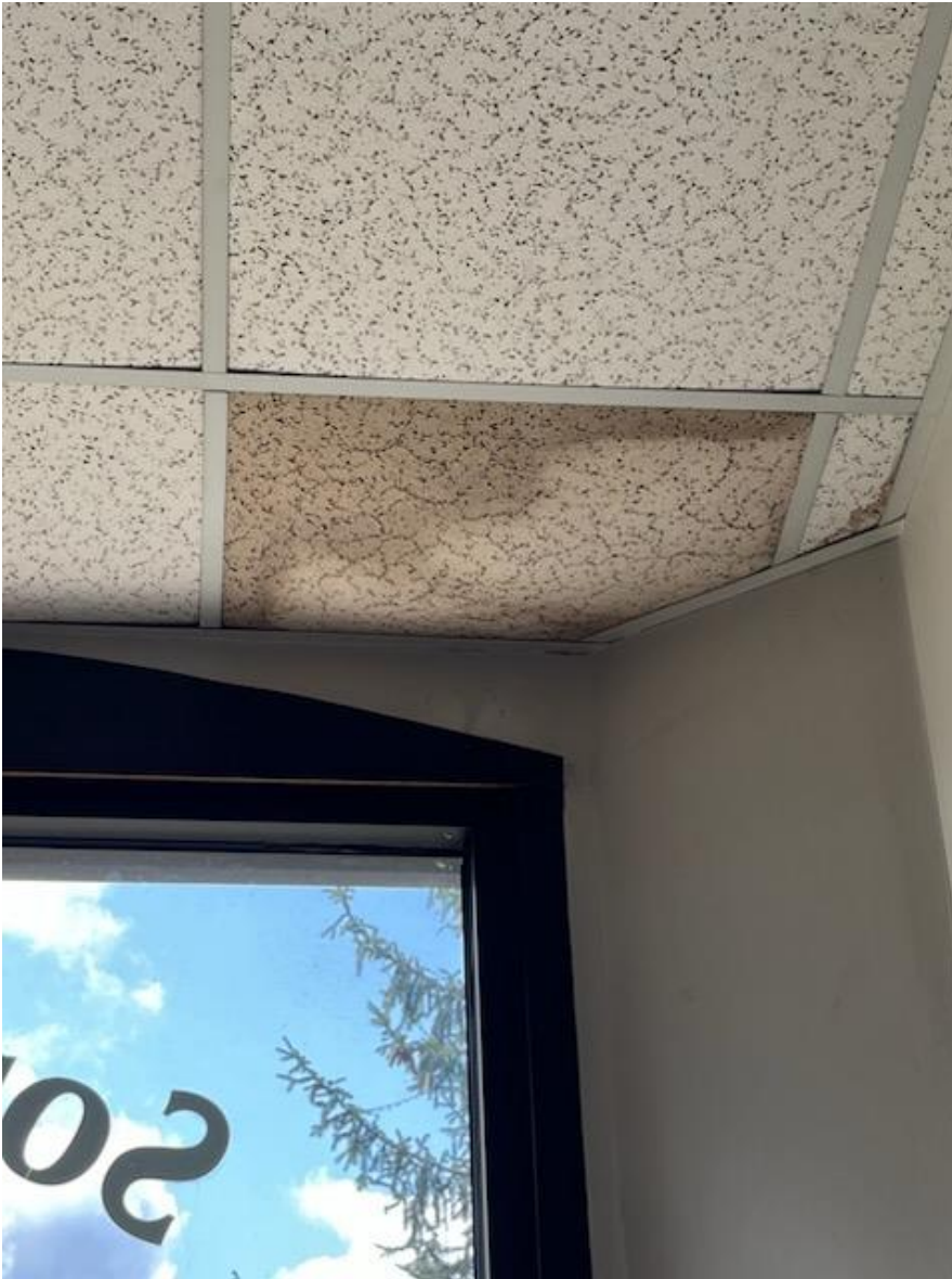
Front Entry Way, has the worst leak, with a bowing ceiling tile.
