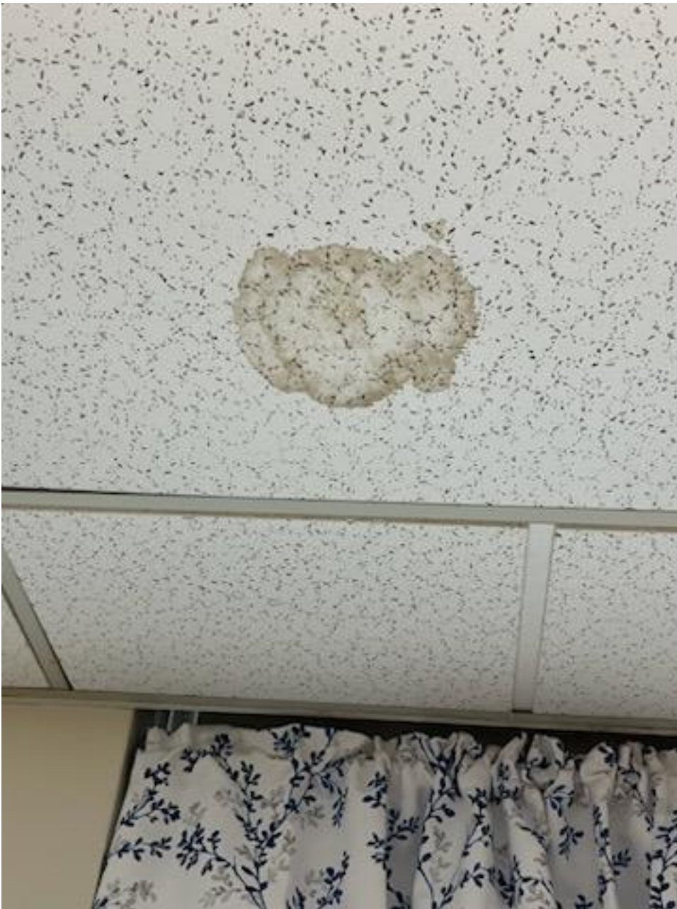
The Finance Office has an active leak.
