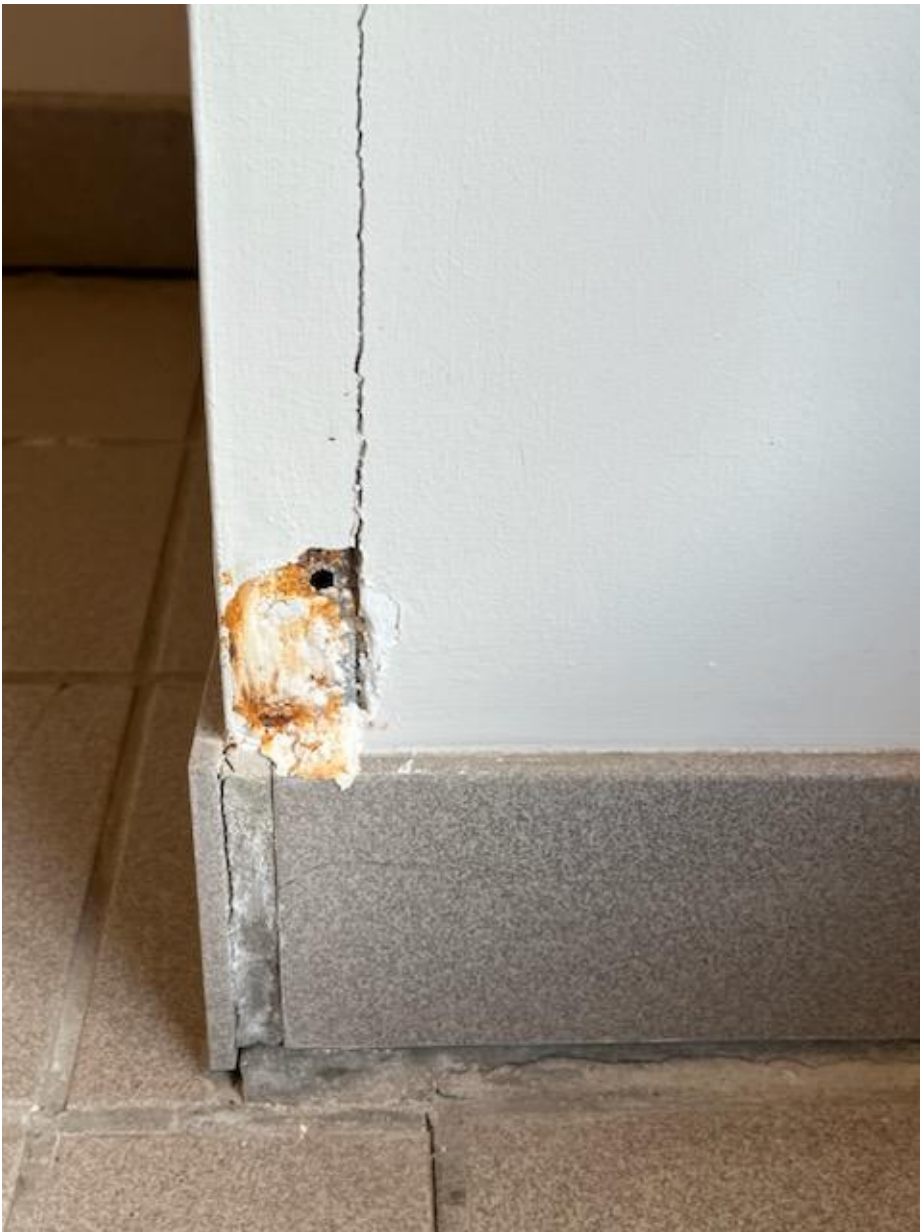
Back, Main entrance door also showing active water leak.
