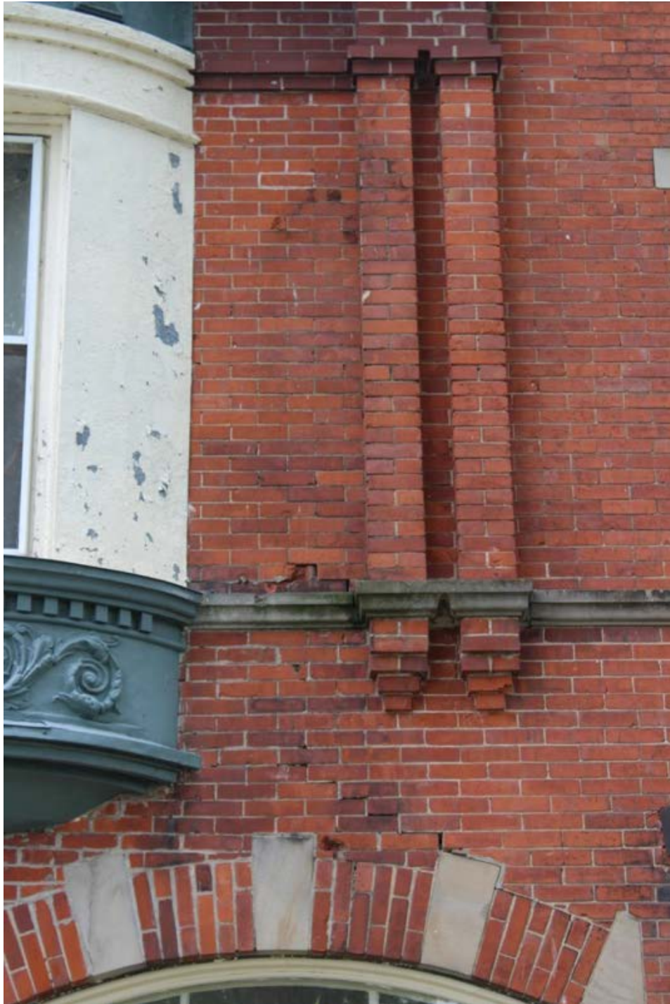
Image 6 Deteriorated brick on south end of façade, looking west. Visible cracking in the mortar joints where mortar is missing and could have water penetration from the inside impacting the brick. Some brick has spalled from the façade where likely water has located behind the wall cavity or incompatible mortar has been placed in the joint. The discoloration of the stone has lichen-like appearance of moisture growth on the belt course of limestone.
