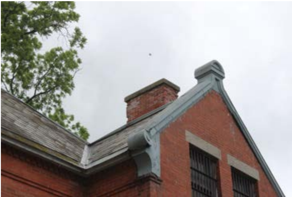
Image 20 Looking southwest at the parapet of the north elevation. Moss and other lichen are visible on the face of the slate roof tiles. Paint has delaminated with peeling at the gable trim and molding. Mortar patching is visible on the east elevation of the chimney. Water has entered areas of the molding and trim
