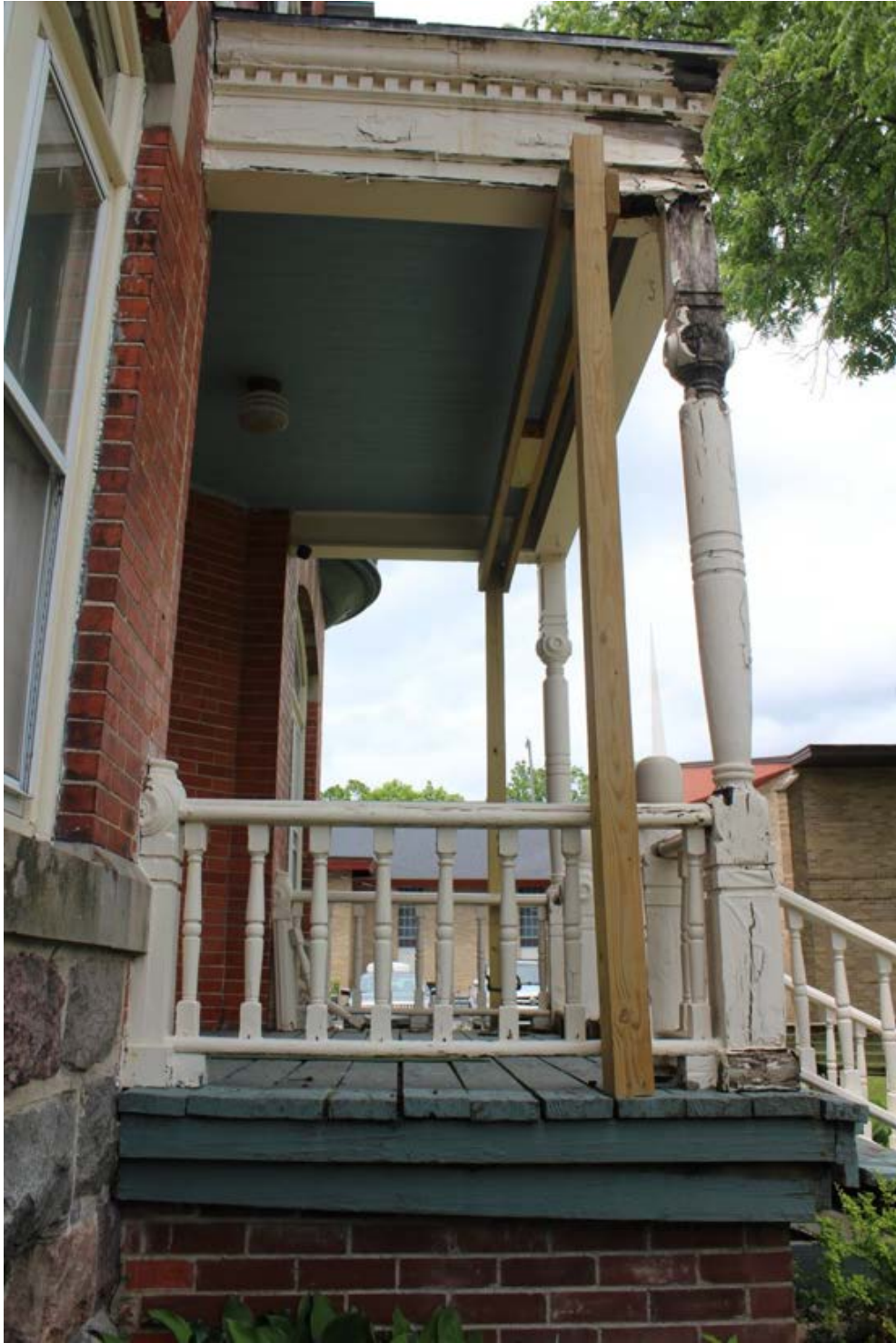
Image 10 View of entryway porch held up by wooden supports, looking north. The portico on the façade has significant damage to due water entering the portico from vacancies/voids and vegetation against the floorboards and foundation of the structure. The two, front columns show wood rot and damage. The porch is later than the original structure. The decorative portico appears to be original, but the columns, flooring, and balustrade are later features. The porch needs immediate attention before further deterioration occurs.
