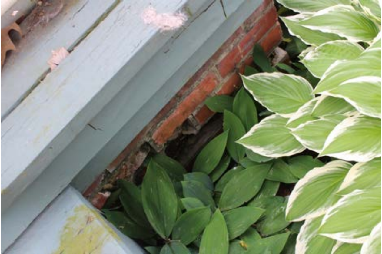
Image 12 Deteriorated brick and mortar underneath north side of porch, looking west. Brick around the porch is deteriorated due to water and moisture against the brick which is causing spalling of the fire skin exterior on the brick. This is problematic. We want to keep water and vegetation away from brick. Mortar joints show discoloration due to lichen, moss, biological growth against the masonry.
