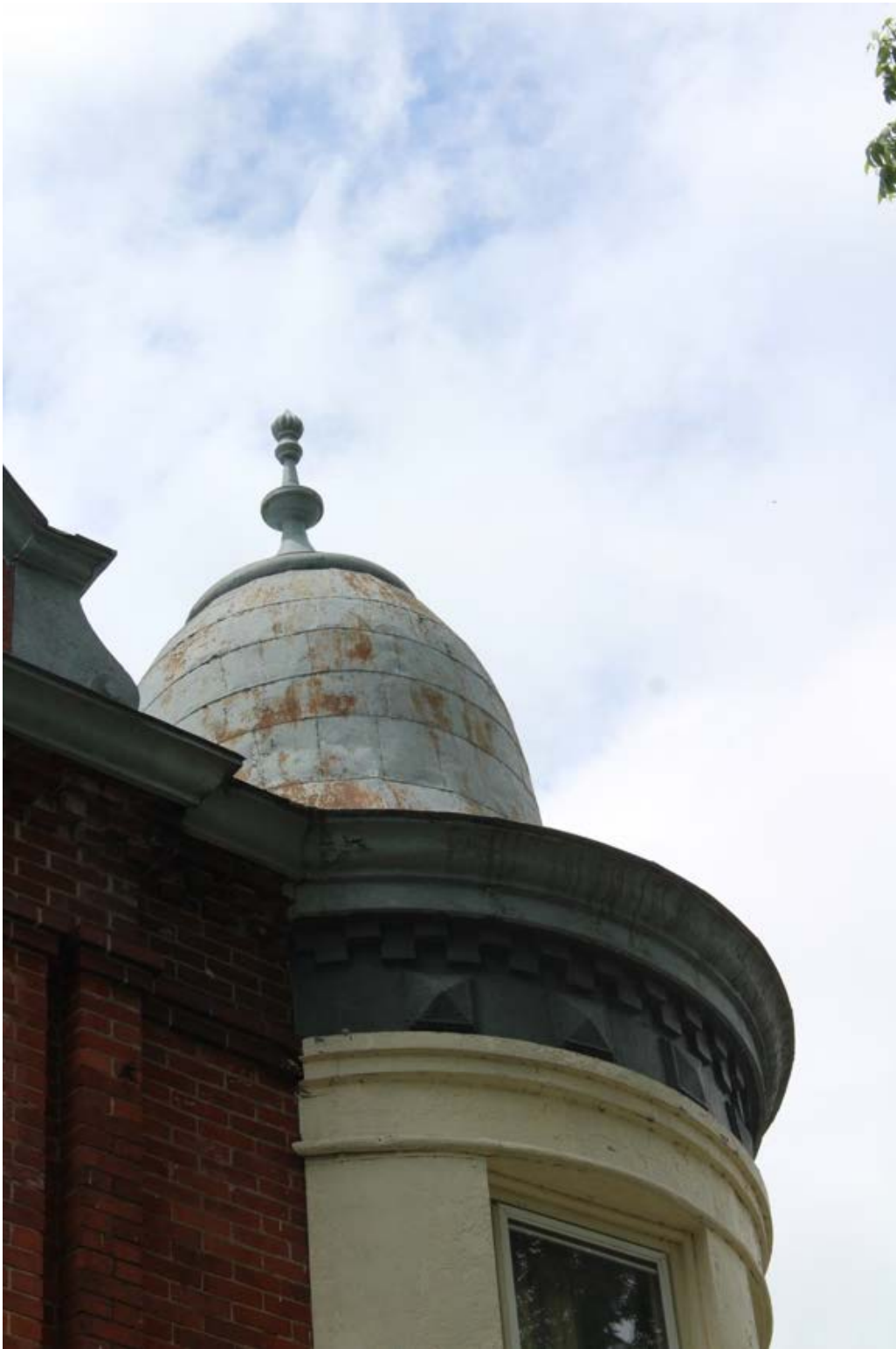
Image 8 View of north turret and its rusted dome, looking northwest Rust and water markings on the rim of the dome show that water is penetrating the dome. The dome appears to be in good condition despite the water infiltration and cosmetic issues.
