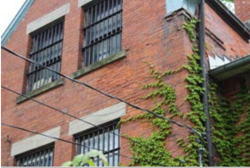
Image 19 Looking south at a detail view of the north elevation at the second and third story. Note the windowsill at the third story has discoloration from vegetation and moisture penetration. Brick below the windows has spalled in areas where the fire skin has spalled off the brick. Vines grow against the upper portion of the elevation.
