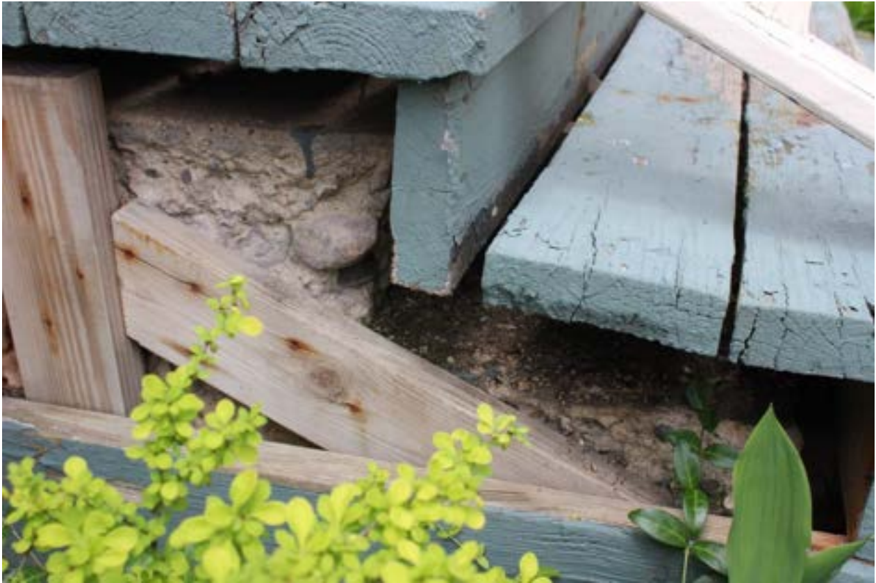
Image 11 View underneath porch staircase to find original stone staircase, looking north. The original structure boasted an aggregate mix for risers and treads. Later, wood boards were added which show visible signs of water damage, wear, and deterioration from vegetation growth.
