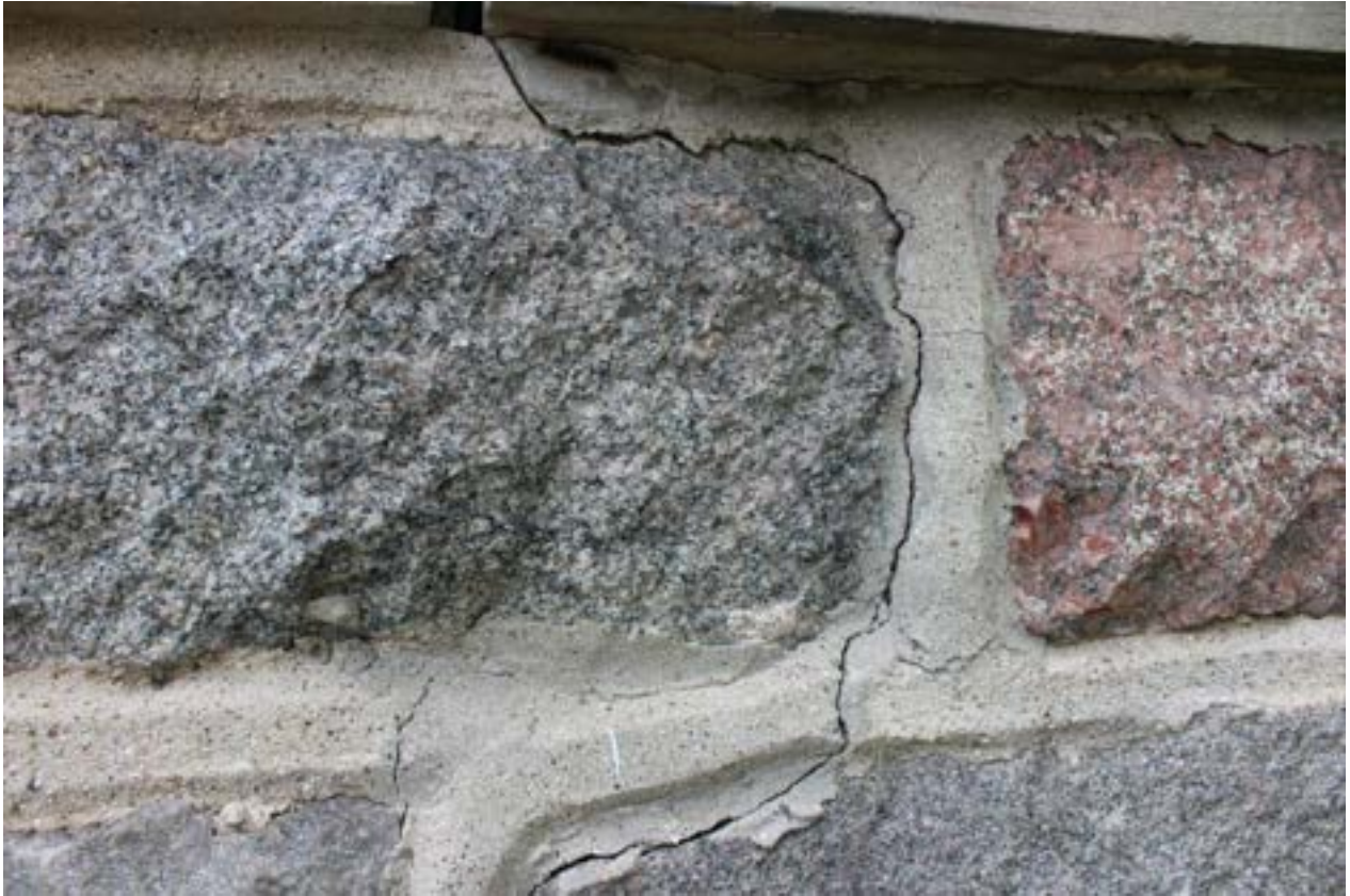
Image 13 Stone foundation on south side of façade and its cracking replacement mortar, looking west. Small, expansion and tensile cracks in the mortar along the foundation.
