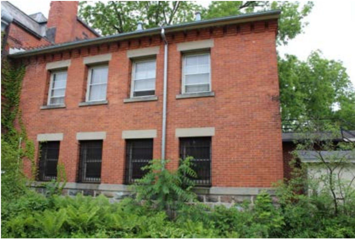
Image 17 The northwest section of the west elevation shows small trees, ivy, ferns, and other biological growth that has spread across this elevation. Vegetation against masonry creates a vehicle for moisture to penetrate brick, stone, and mortar joints.
