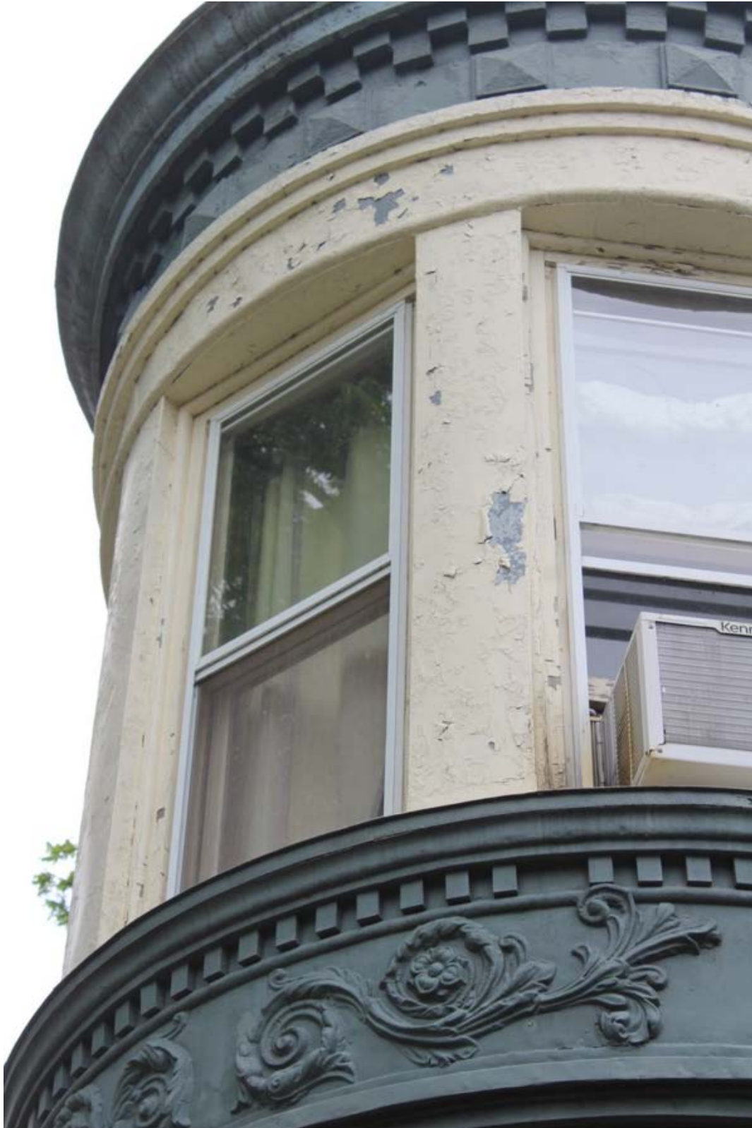
Image 7 Close-up of south turret and its exposed metal material, looking west. Paint failure is visible where paint is peeling and has delaminated from its surface. Rust and water markings on the rim of the dome show that water is penetrating the dome.
