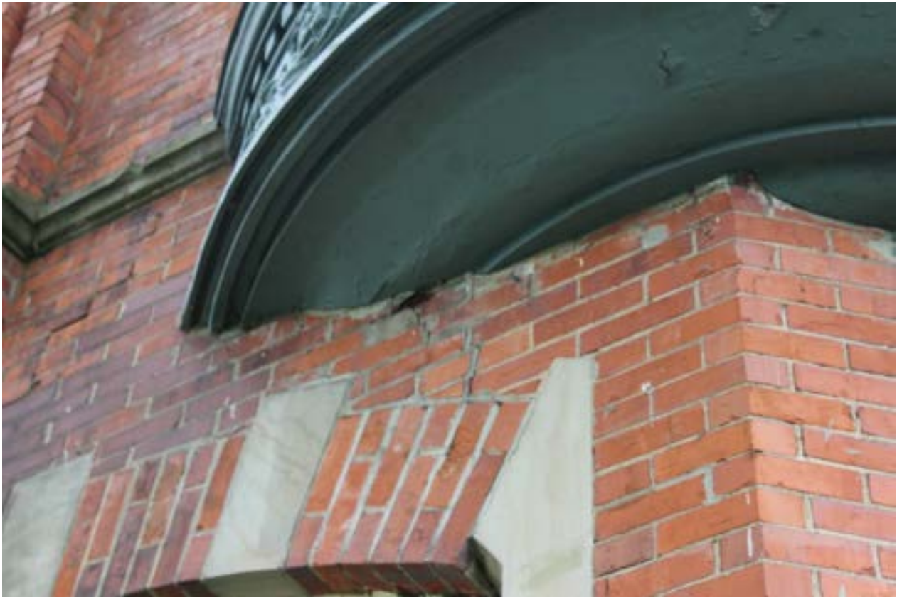
Image 9 View of intersection between north turret and façade brick, looking west. There appears to be mortar that has been inserted in patching locations across the structure. This mortar appears to be a different aggregate mix than the original “mother” mortar mix. This mortar can be stronger than the brick itself and jeopardize the ability for the brick to have an expansion and contraction when temperatures change.
