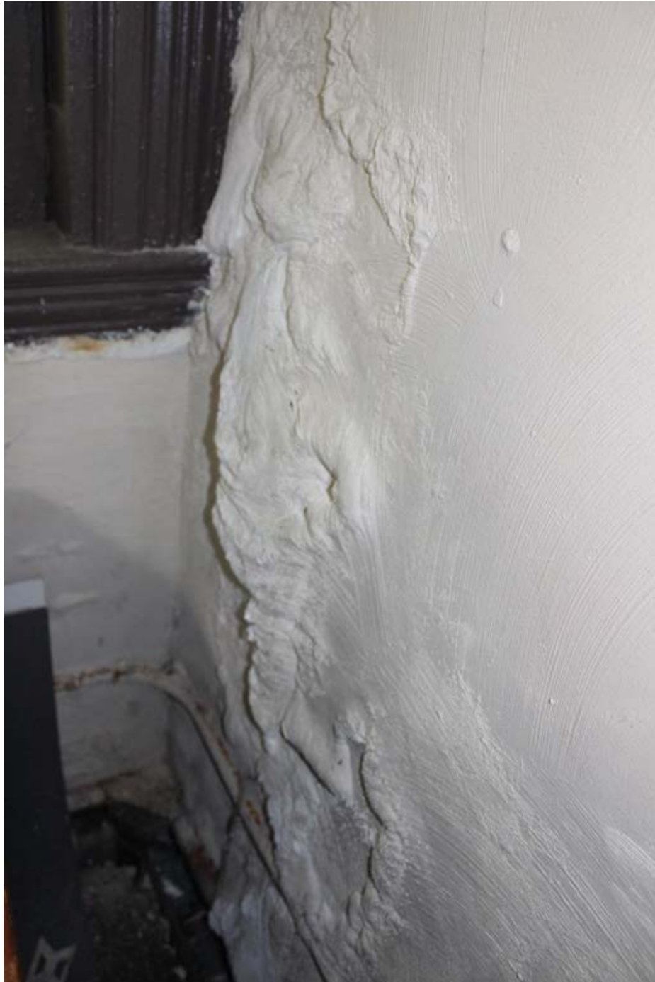
Image 36 Northwest corner of the wall on the first floor of the jail kit house where water has penetrated within the interior of the wall and has resulted in plaster deterioration. Electrical line is rusting along wall from water penetration.
