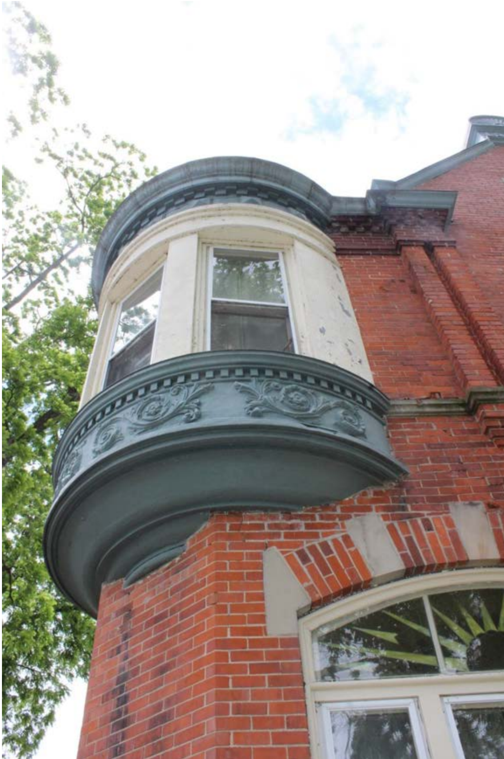
Image 5 South turret on façade, looking west. Brick discoloration is occurring from water infiltration in brick where water is being channeled down the brick due to lack of water (gutter) removal system. Paint is peeling on the turrets. Also, rust is visible on the dome above the turret. Some caulking issues around the turrets and windows that create small fractures in the brick.
