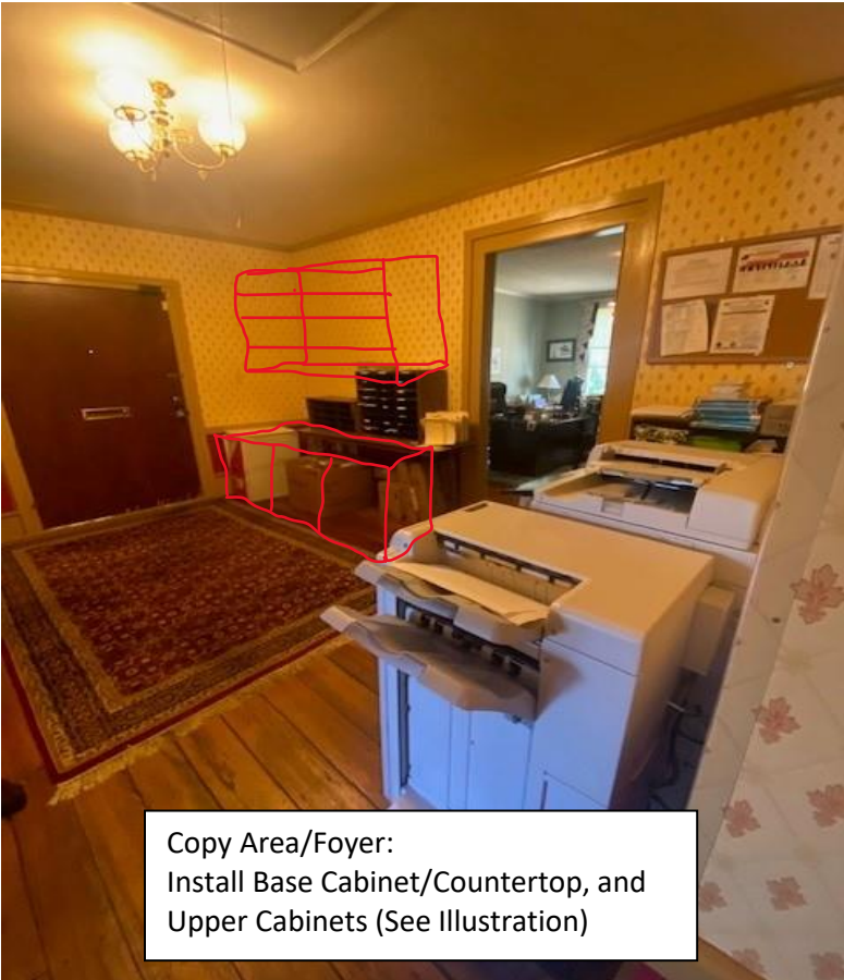
Existing Kitchen (Future Office): Remove Cabinets, Appliances, Remove Wallpaper, Prep/Paint Walls, Trim and Window
