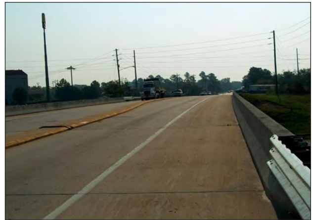
Today the Blythewood Road/I-77 overpass is not pedestrian friendly and lacks even basic sidewalks
