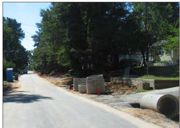
Studies should be undertaken to evaluate expansion of existing water and sewer infrastructure
