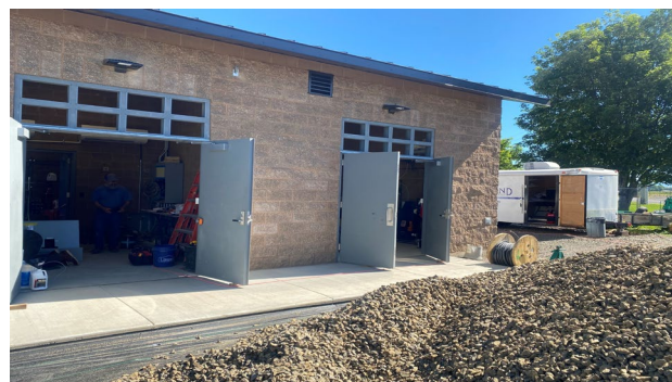
Well #4, one of two new sources that we have been developing, has now been completed! Development of Well #6 is underway!
