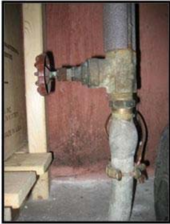
Lead service lines often have a "bulb" shaped connection
