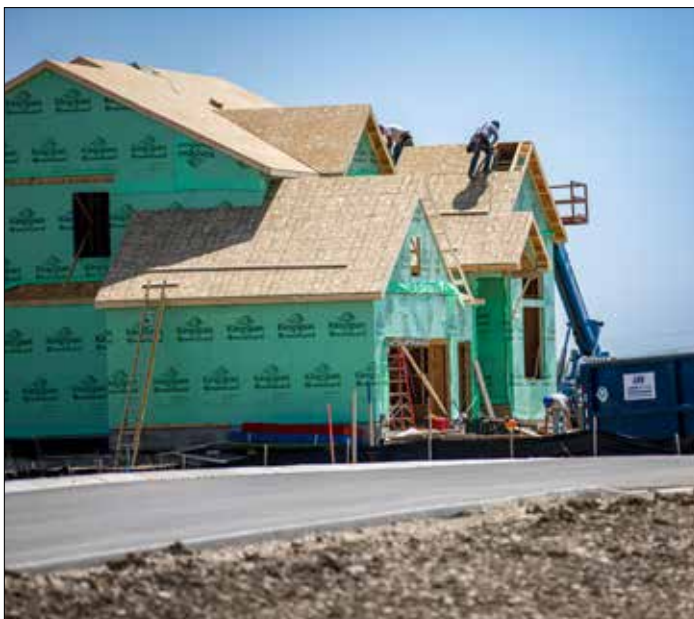
Work continues at Talamore, a Lennar-built resort style community in Huntley that will feature a variety of homes and amenities.
