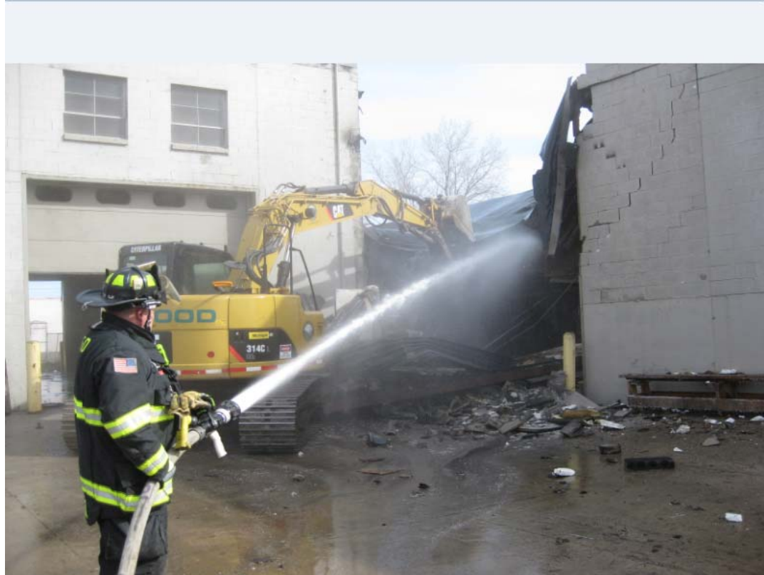
3060 Breton - March 24th Fire and Public Works Departments work together to put out the fire
