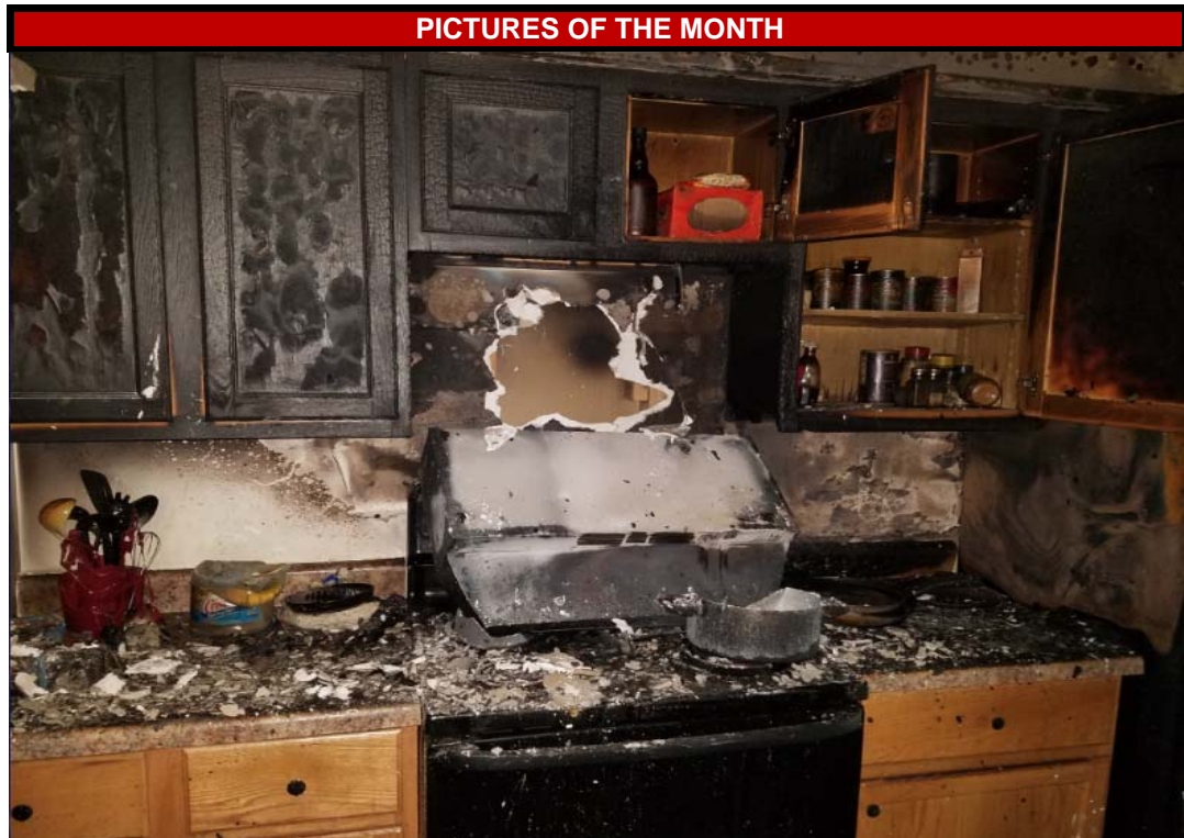
Fire fighters rescued two residents from this 44th St. apartment early in the morning on September 22nd. One succumbed to injuries on October 9th.
