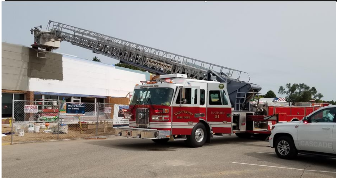
6455 28th St., SE - 9/14/20 Assisted Cascade with fire in multi-tenant building being renovated
