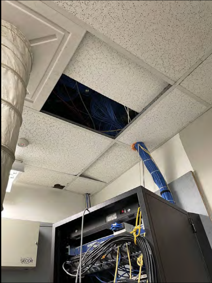
Ceiling tiles missing; fire wall penetrations
