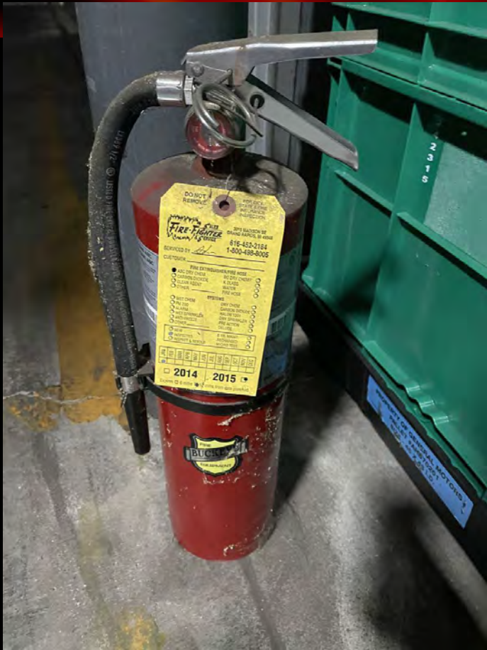
Extinguishers not mounted properly and/or out of date
