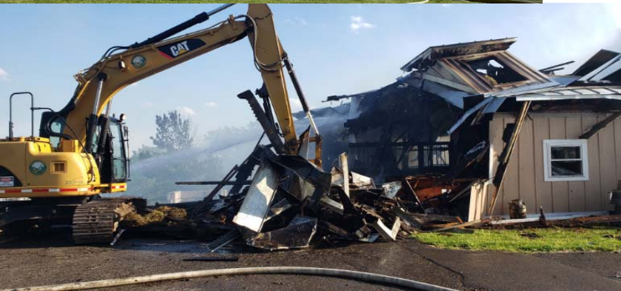
Ultimately DPW brought down the building so hot spots could be extinguished.
