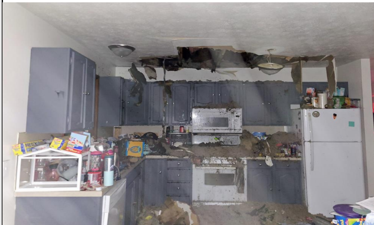
Kalamazoo Ave., May 12, 2023 - vent fan above ceiling
