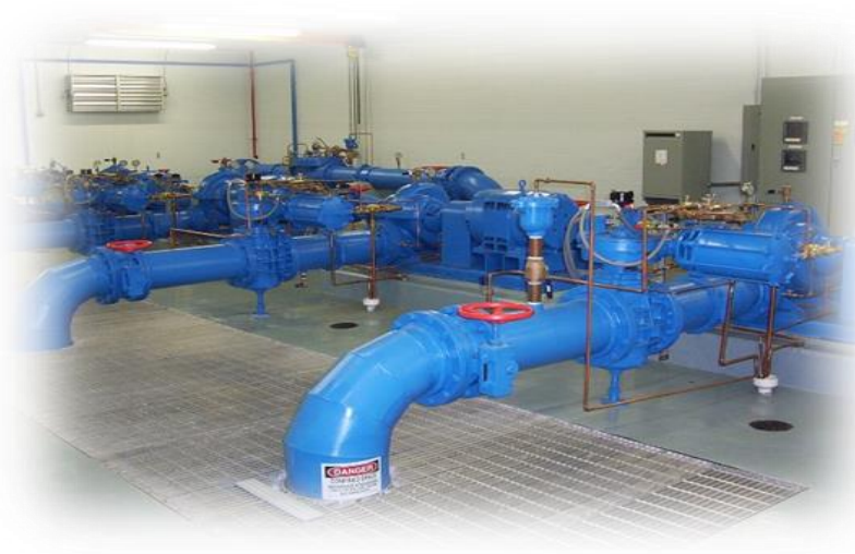
City of Kentwood Water Pumping Station
