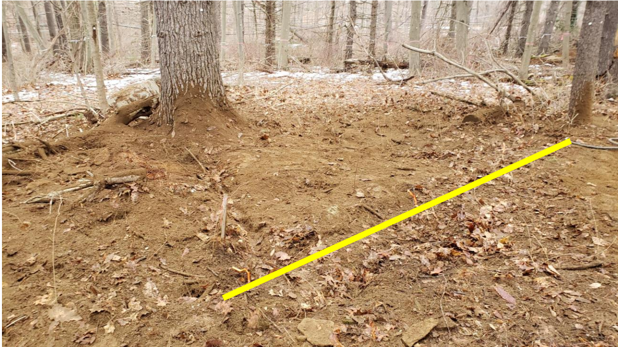
Photo showing the marked limits of where excavation can occur (yellow line). If excavation or grade change is needed between the tree and this line, the tree should be removed.
