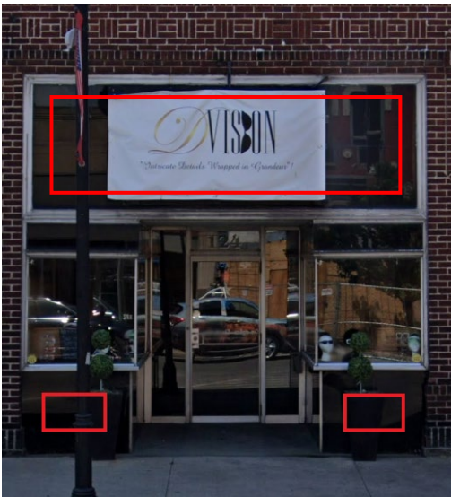
Decorative molding locations (approx.)
