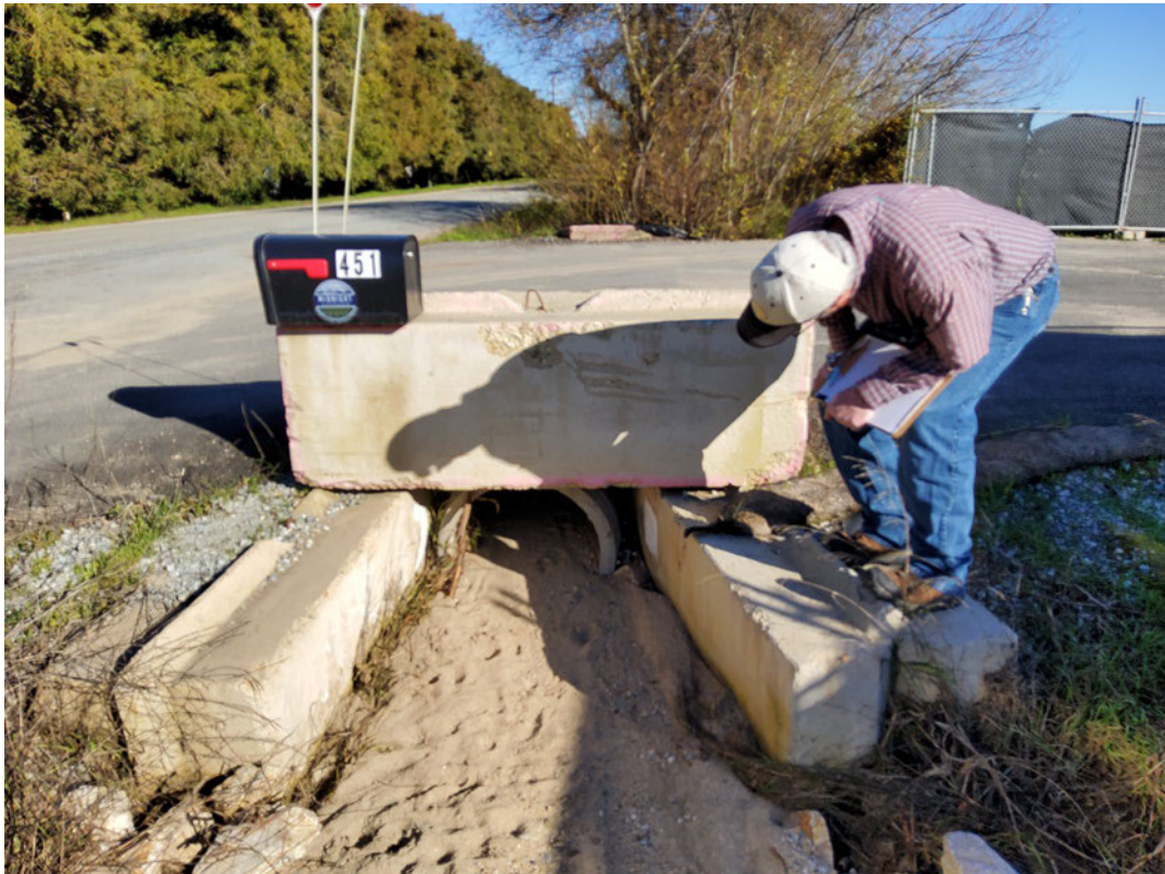
48-inch Culvert Sediment Impact
