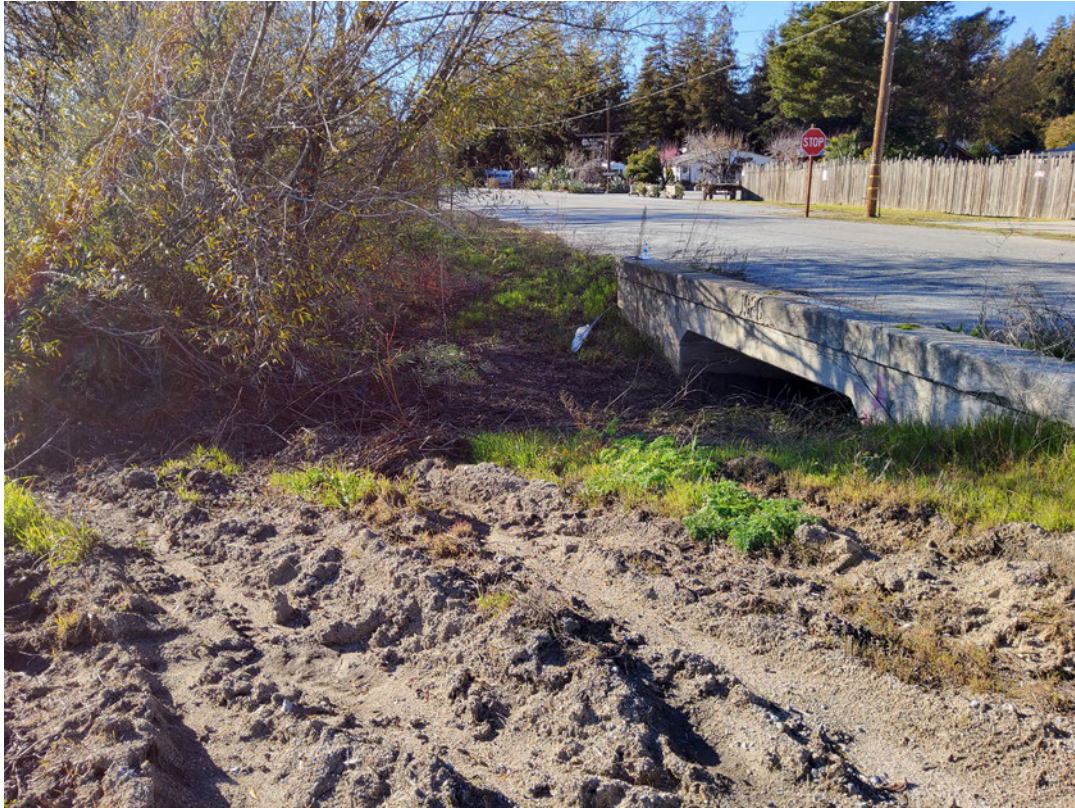
Box Culvert Sediment Impact
