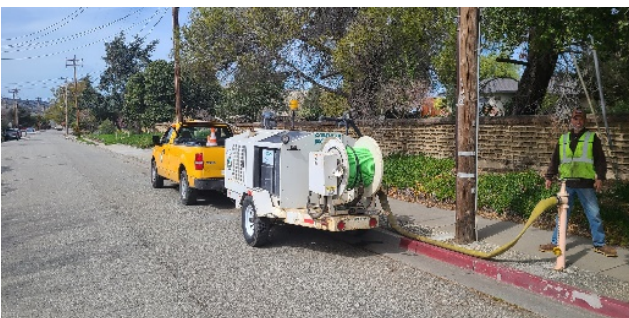
Gil our Public Works lead collection system worker filling up hydro flushing Trailer.
