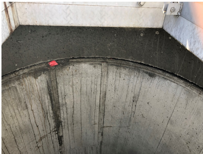
Figure 5 – Possible Signs Of Infiltration Through The Concrete Joints
