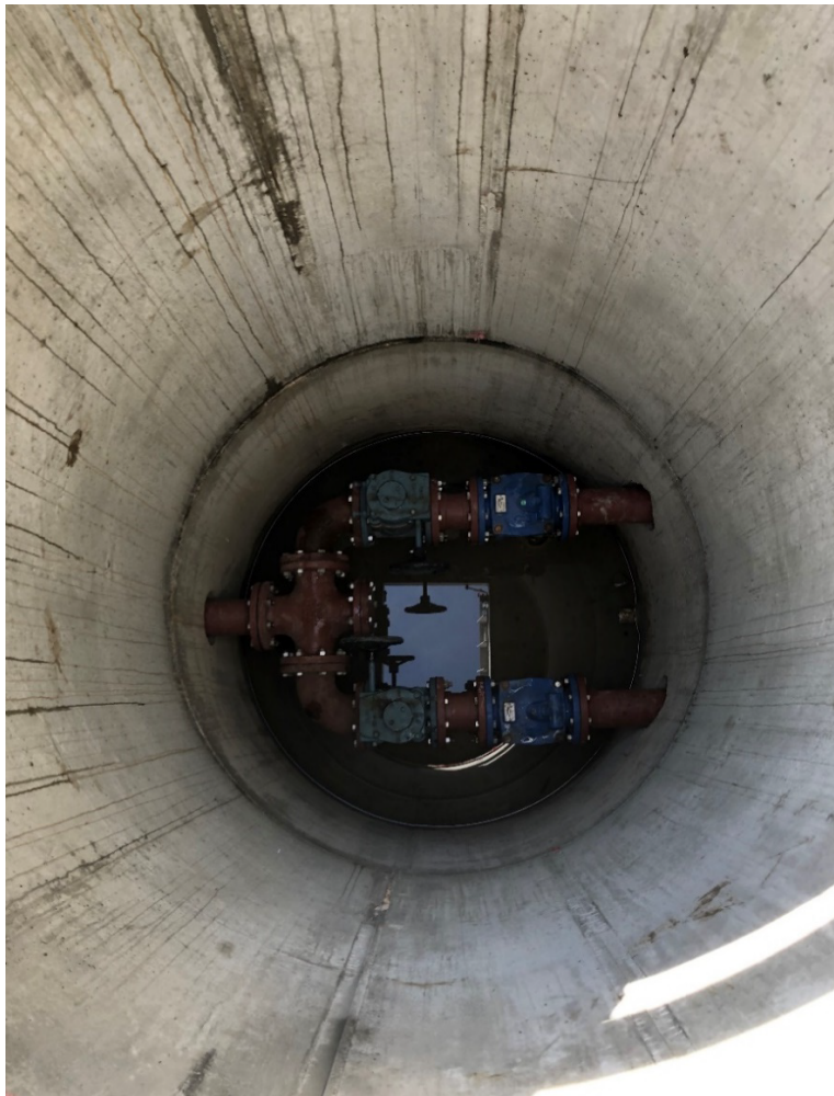
Figure 4 – RVSLS Valve Vault With Standing Water
