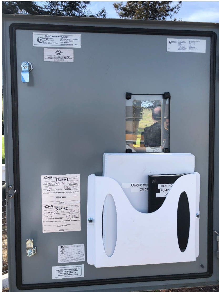
Figure B.1 – Inside Door Of Control Panel
