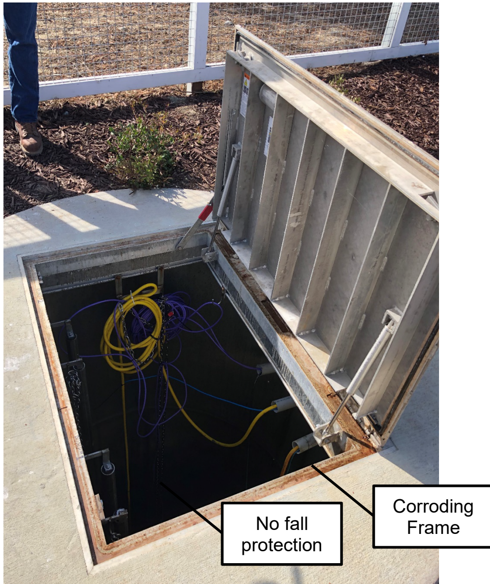
Figure 2 – RVSLs Wet Well Access Hatch
