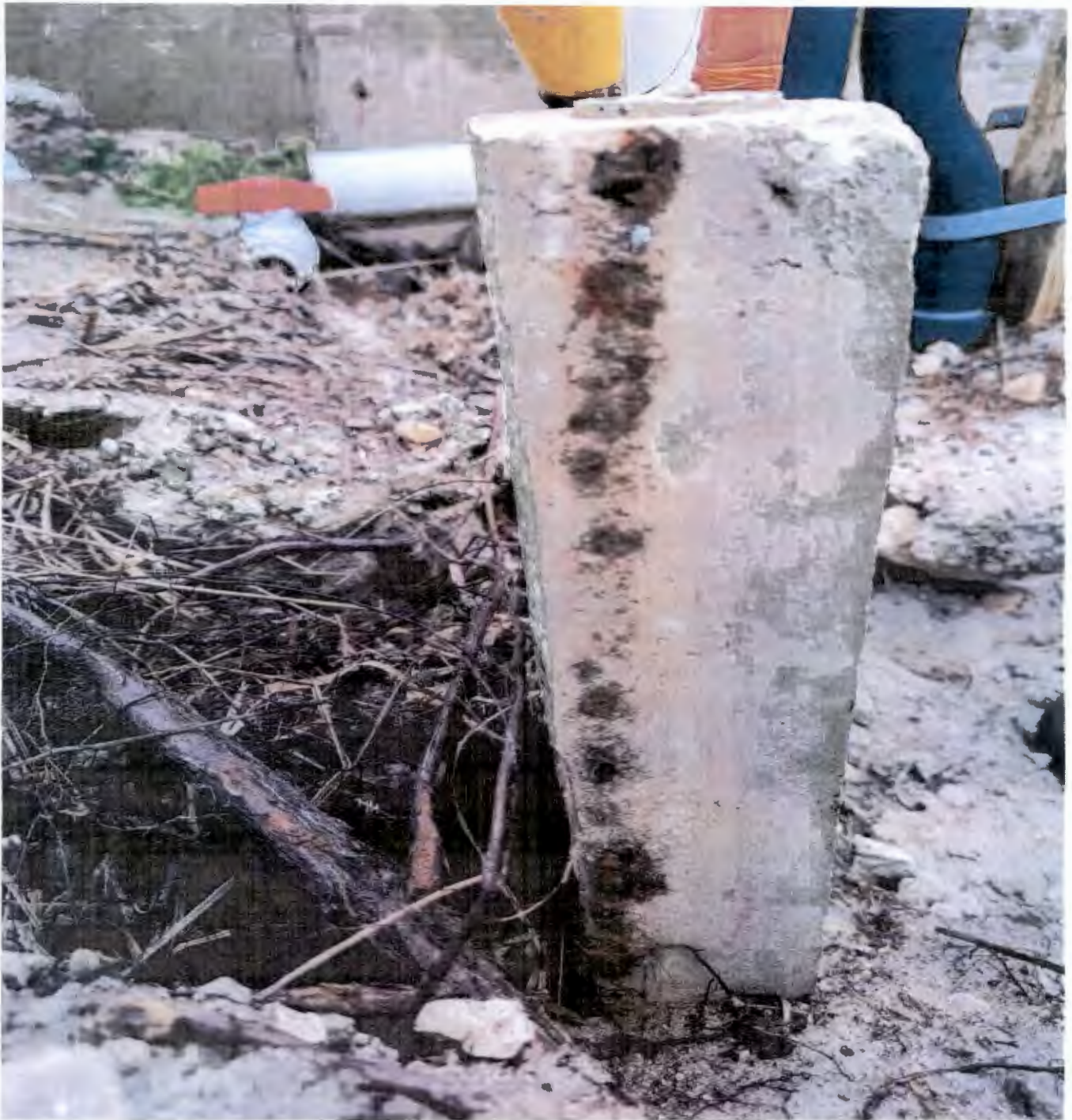
Rust on concrete monument is constant with rebar found lying beside the concrete monument.
