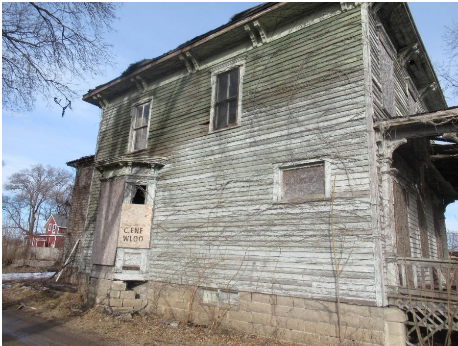
(West side of the house, with fallen foundation)
