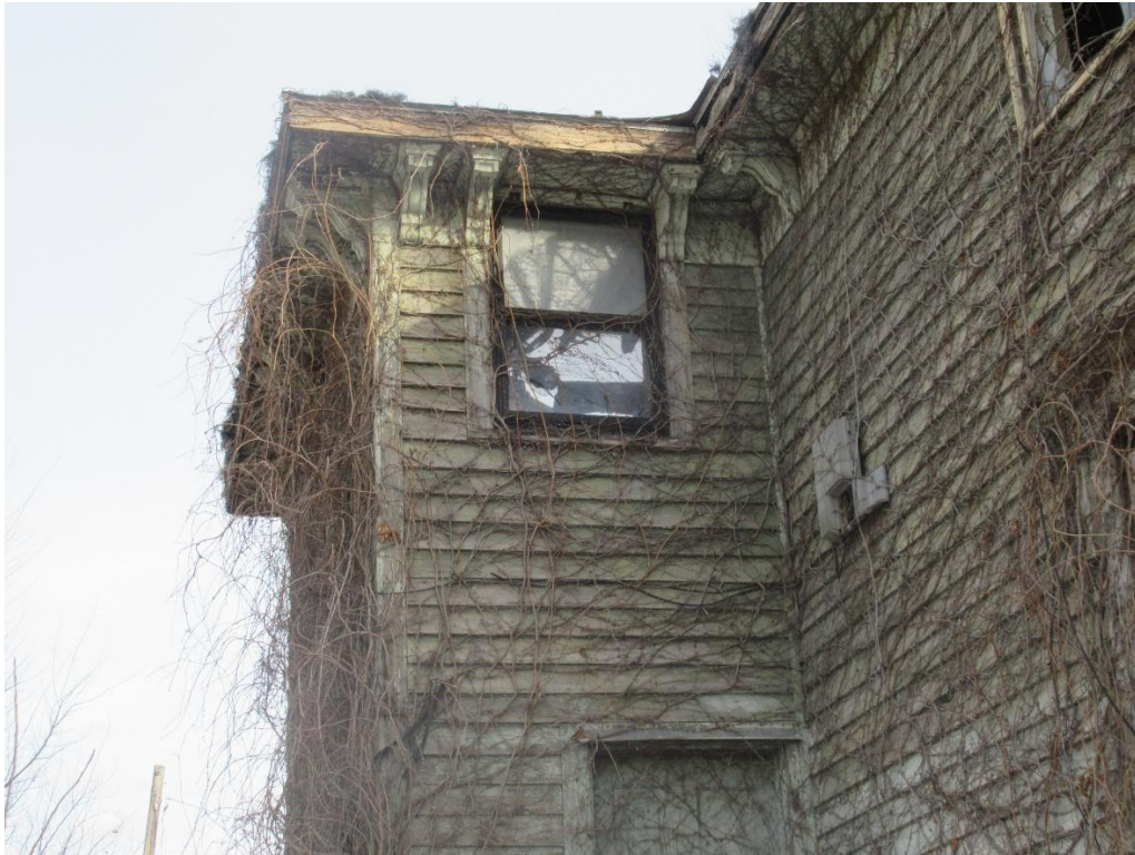
(Looking at a hole in the roof through a window)
