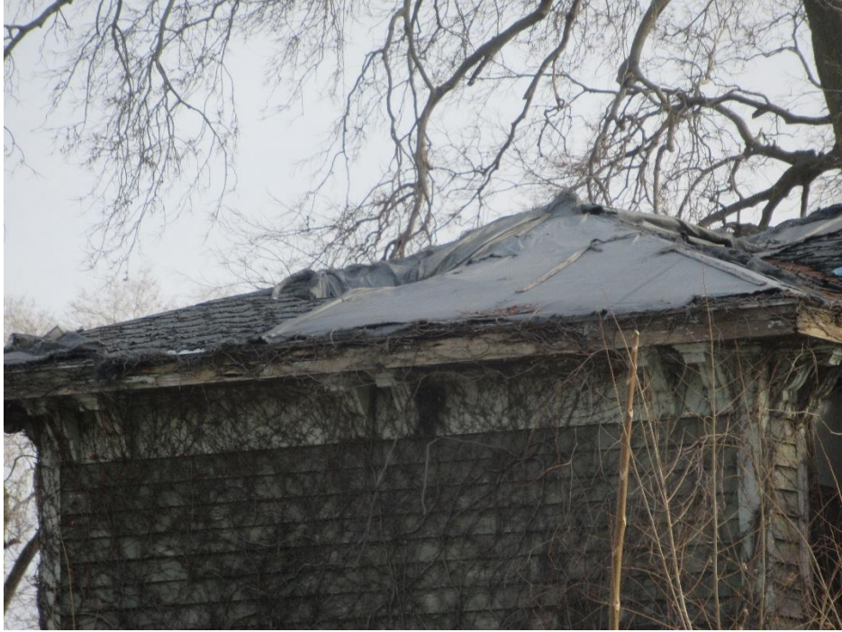
(Hole in the roof)
