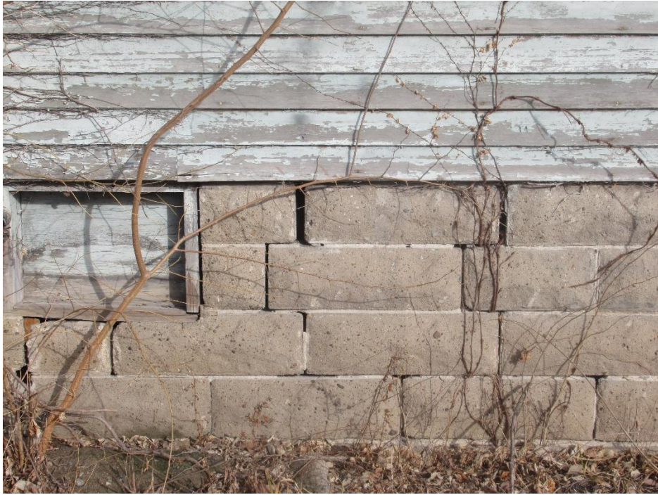
(Problems with the foundation)
