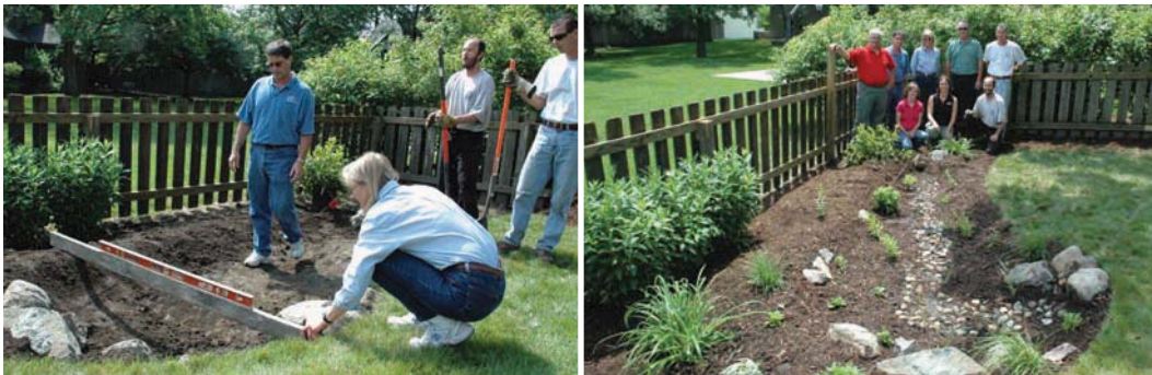
A rain garden is installed at the home of Bob Quinn, host of the "Big Show" on 1040 WHO Radio in Des Moines. Quinn and WHO help promote rain garden installations in Iowa.
