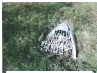
Storm outlet clogged by debris
